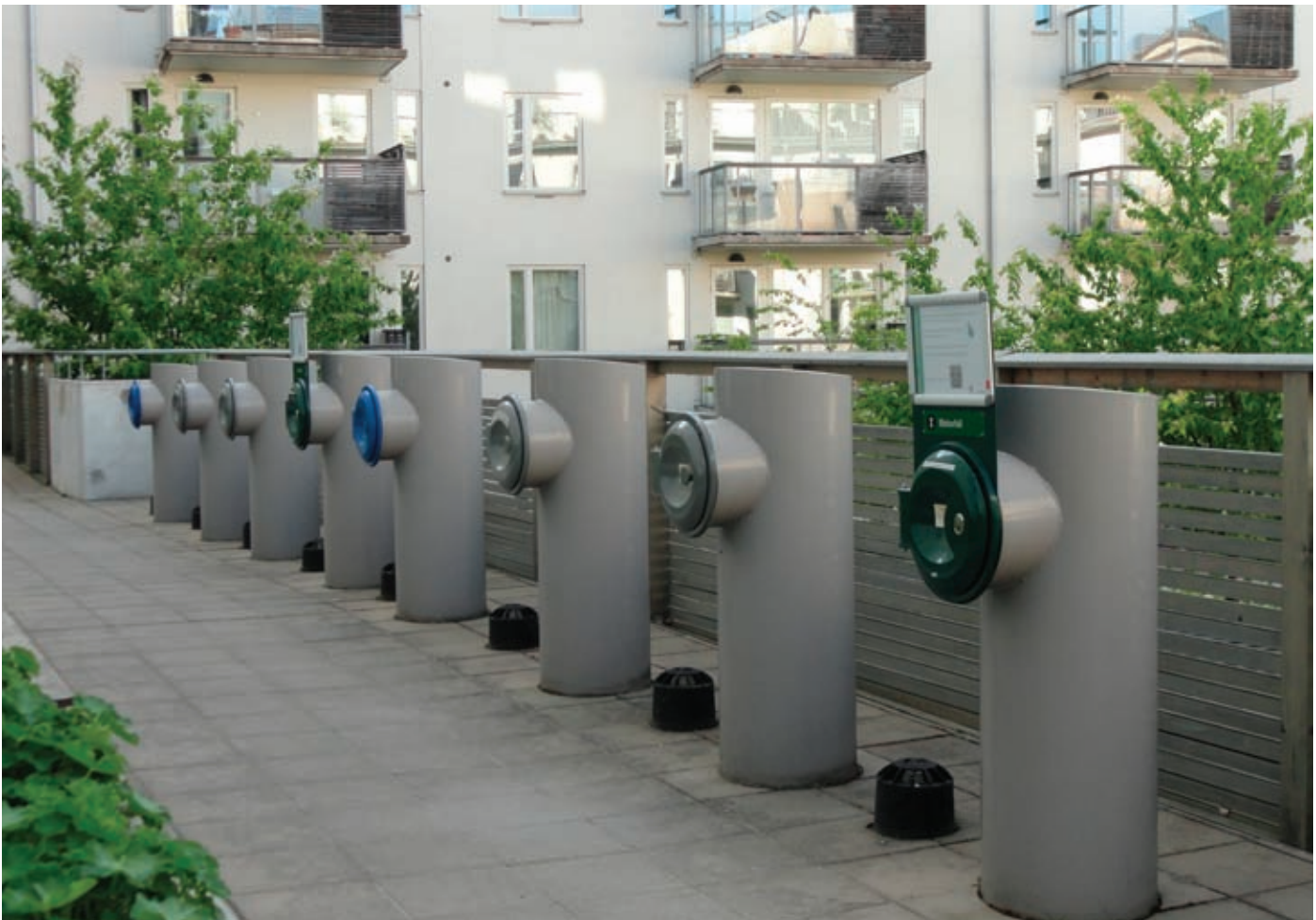
Above: Pneumatic waste collection systems.
